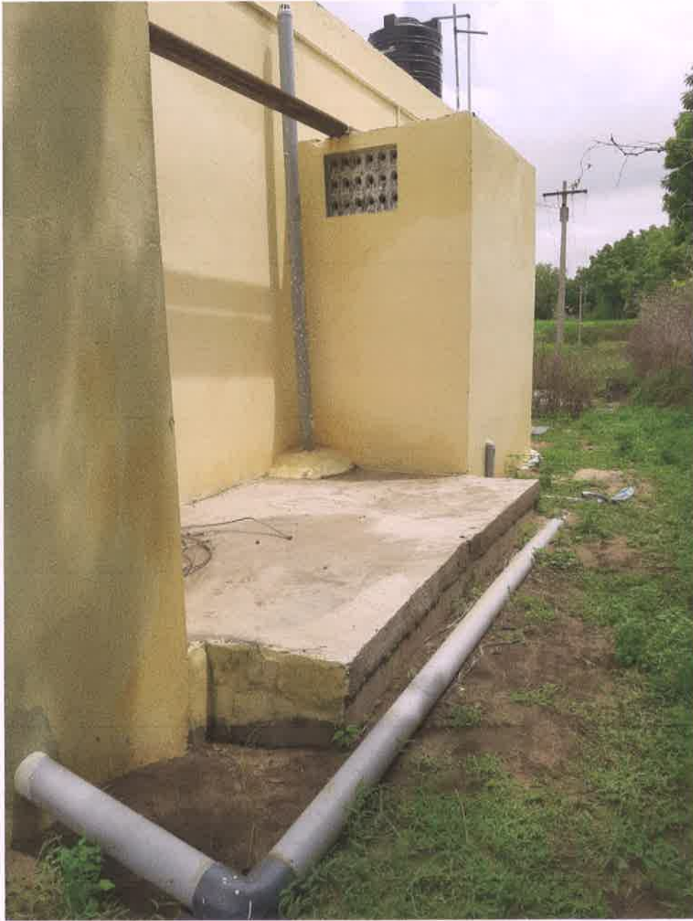
(Septic Tank at Mines Office)
