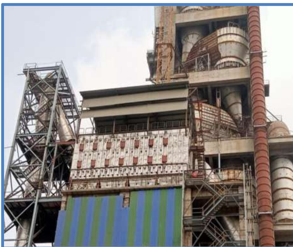
Bag House for Coal Mill
