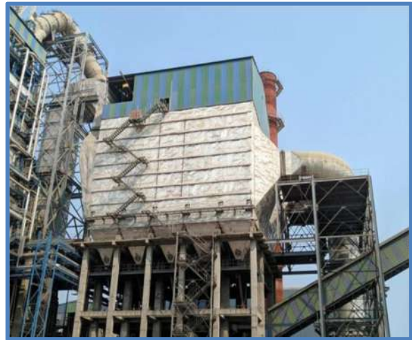
ESP for Clinker Cooler
