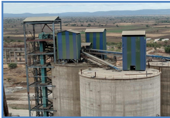
Bag filter at cement silos top
