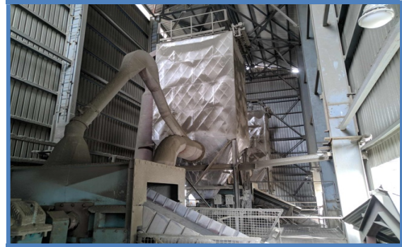
Bag filters at clinker transport system
