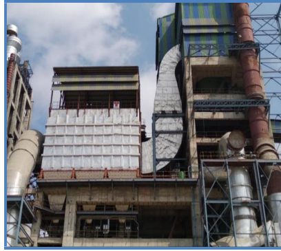
Bag House for Cement Mill
