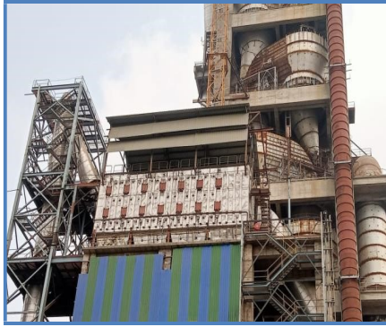
Bag House for Coal Mill
