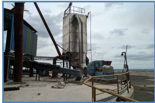
Bag filter at blending silo top
