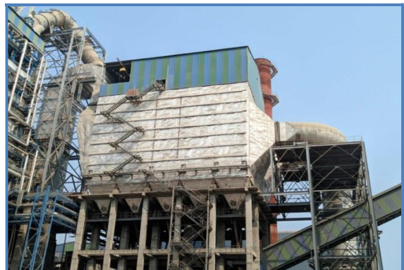
ESP for Clinker Cooler
